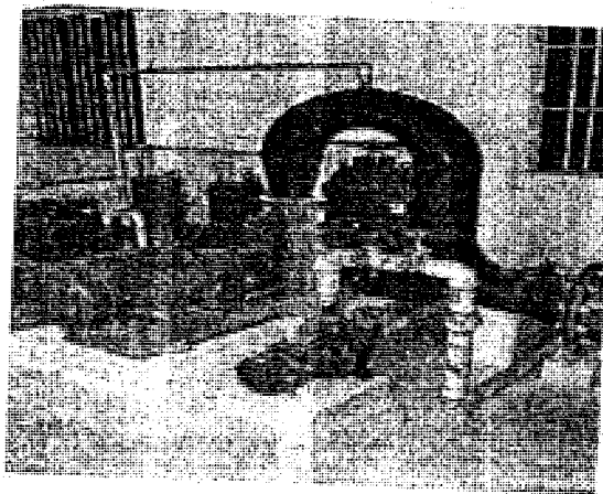
Water pump to chemical house
